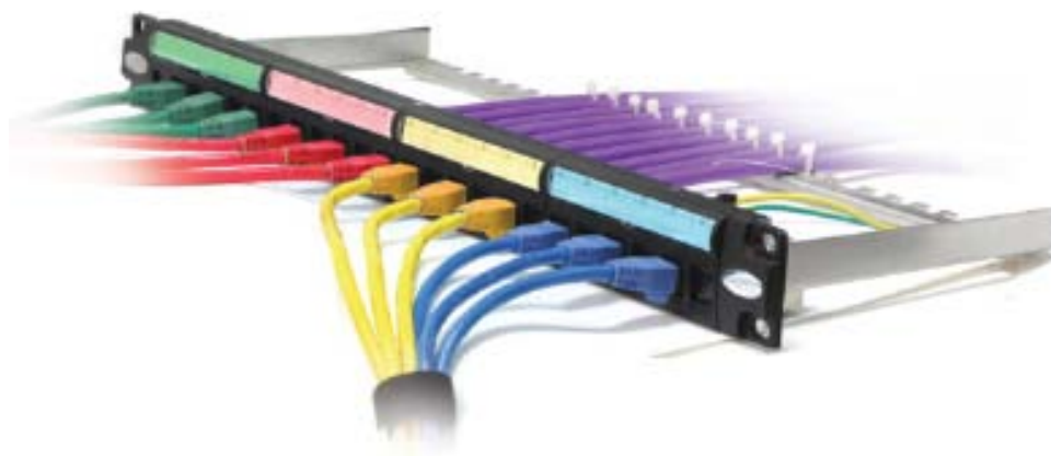
FTP Patch Pannel
